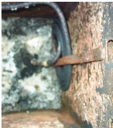
Picture 63 A metal tube coil for steam generation used in a stove
