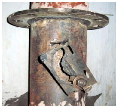
Picture 62 Butterfly valve used in a chimney
