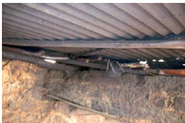
Picture 45 Soot accumulated on the roof of a kitchen
