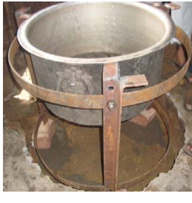
Picture 75 Using an utensil with water (level) for installation of a stove parallel to the ground.
