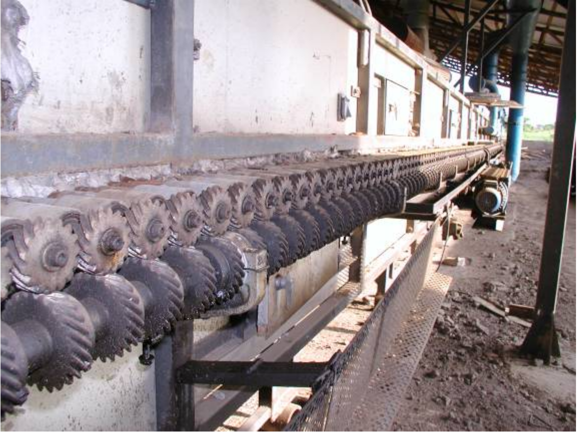
For people with really big ambitions, this Italian made tunnel kiln goes nonstop to produce ceramic floor tiles.
